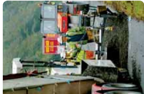
Tarmac is increasingly using recycled materials and energy-efficient processes in its road building activities (see page 51).
