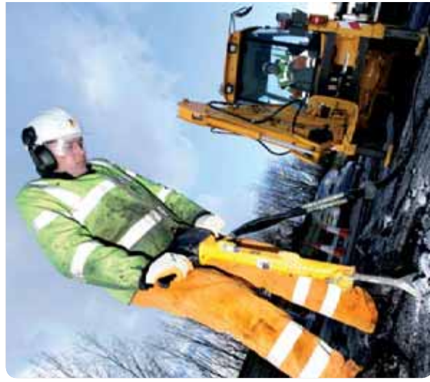
Tarmac is labelling all equipment to help employees calculate and manage their exposure to health hazards. The streammaster, which reduces exposure to HAVS, is being introduced throughout the company.
