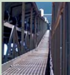
Left: An energy audit identified an opportunity for Namakwa Sands' mineral sands operation in South Africa to reduce energy consumption by changing conveyor belt lights to day-night switches.
