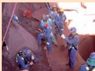
Left: Managers at Kumba’s Sishen iron ore mine identified the potential risk that a worker could fall into the primary crusher during inspections and maintenance. In order to provide proper support during these tasks, a life-line with a roller impact lock-system, similar to car safety belts, has been developed and tested by the South African Bureau of Standards.
