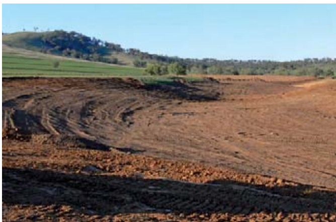
Above: Rehabilitation work is being undertaken to repair the severely eroded Australian Hunter Valley.
